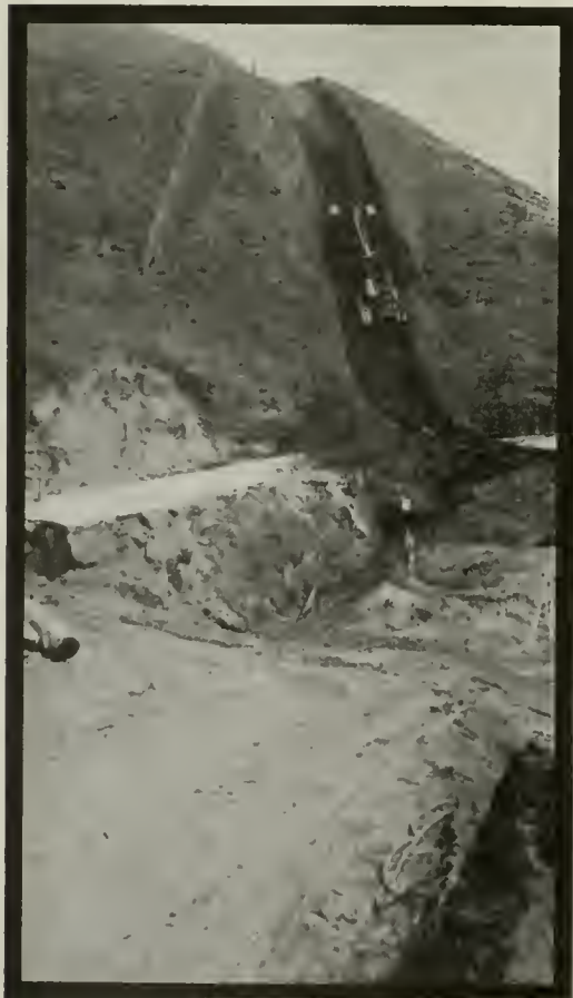
D. McDonald is the contractor on this section of the San Simeon-Carmel highway
